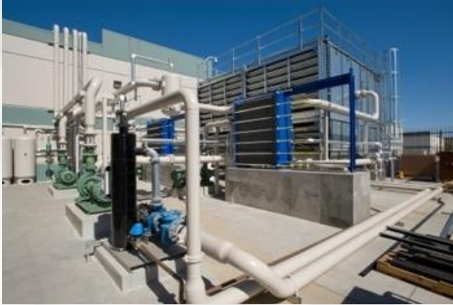
This large condensing unit is 99 feet from a scheduled building, and has a $200K ACV.
