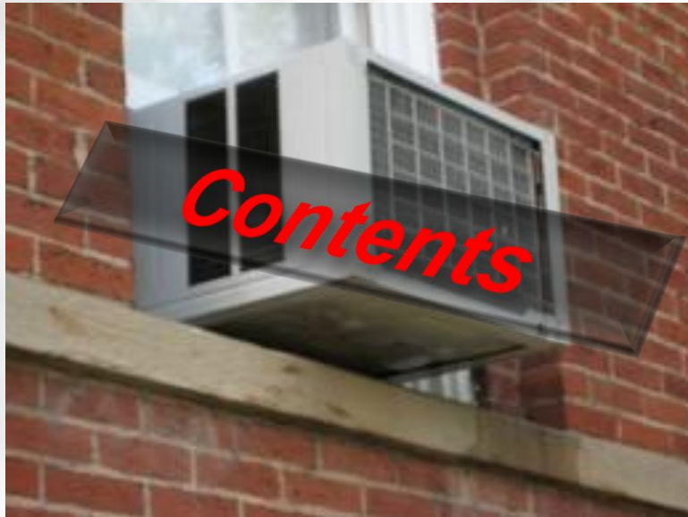
Window HVAC Unit
