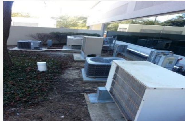
These small condensing units are all within 20 feet of scheduled building; and have ACV's < $50K.
