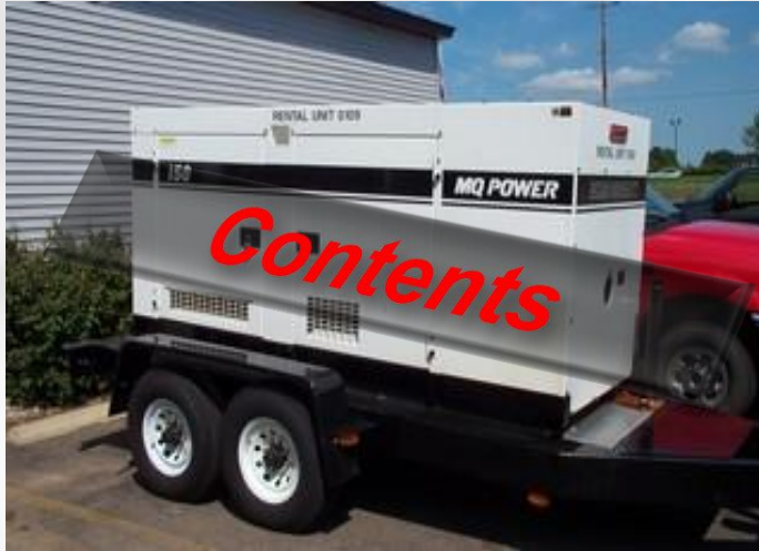
Generator: sitting on a portable flatbed trailer
